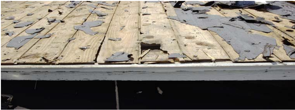
Older Deteriorated and Damaged Deck (Board Decking)
