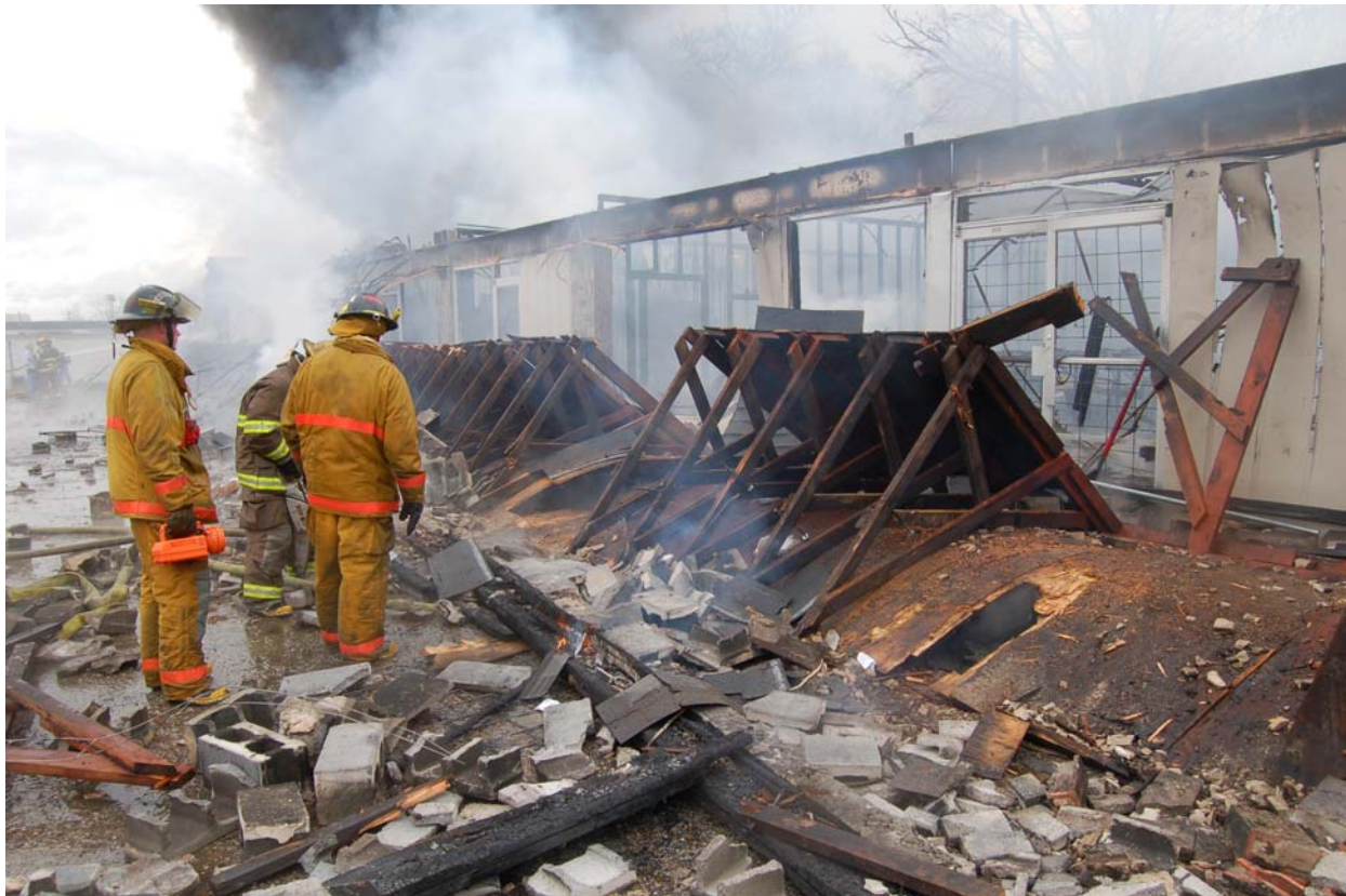
Figure 10. South view of collapse (Photo by Denison FD)
