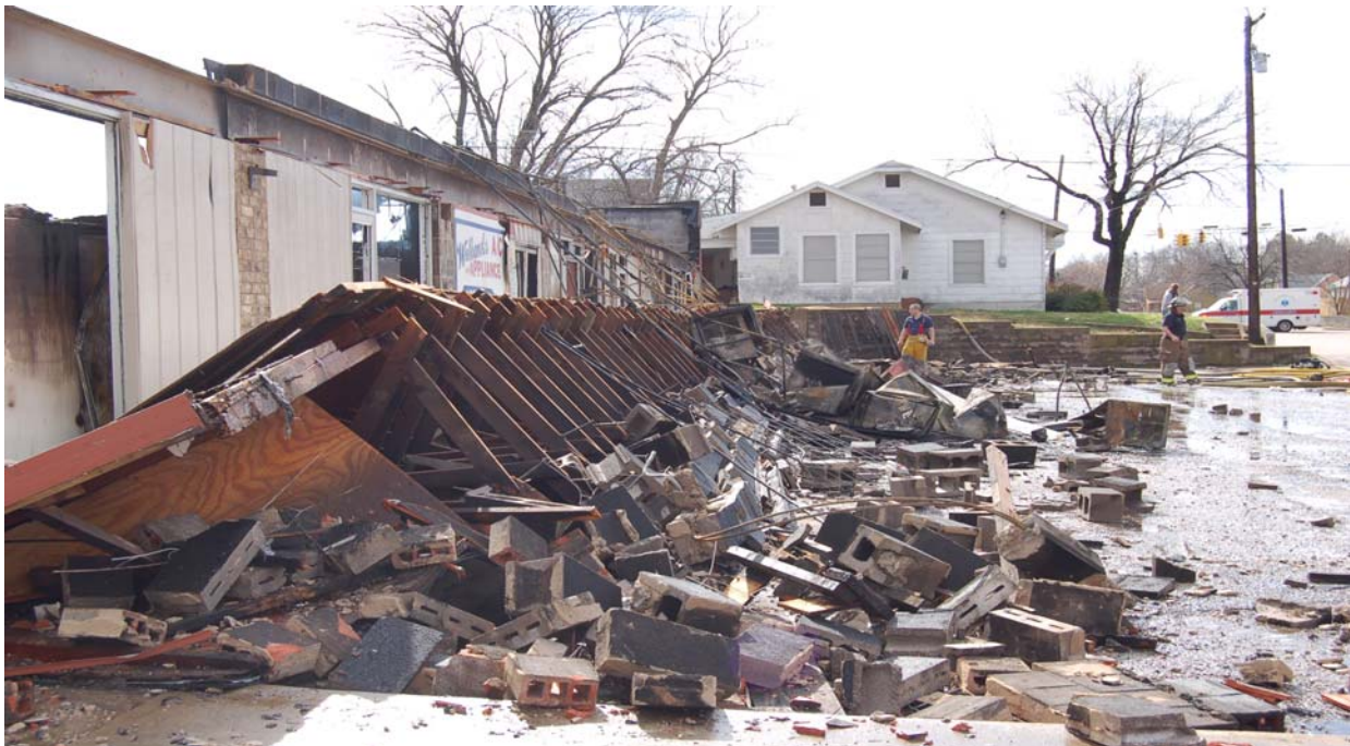
Figure 1. Collapsed awning (Photo by Denison FD)
