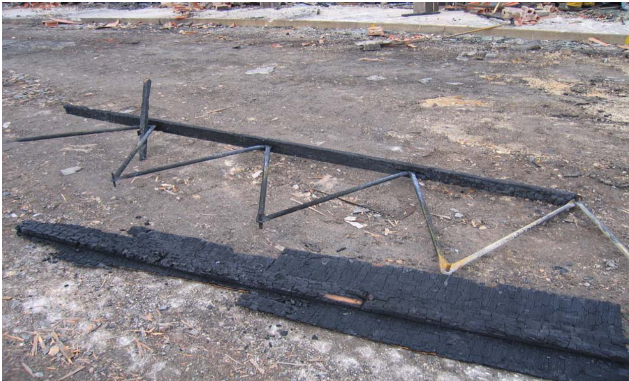
Figure 4. Remains of truss (Photo by SFMO)
