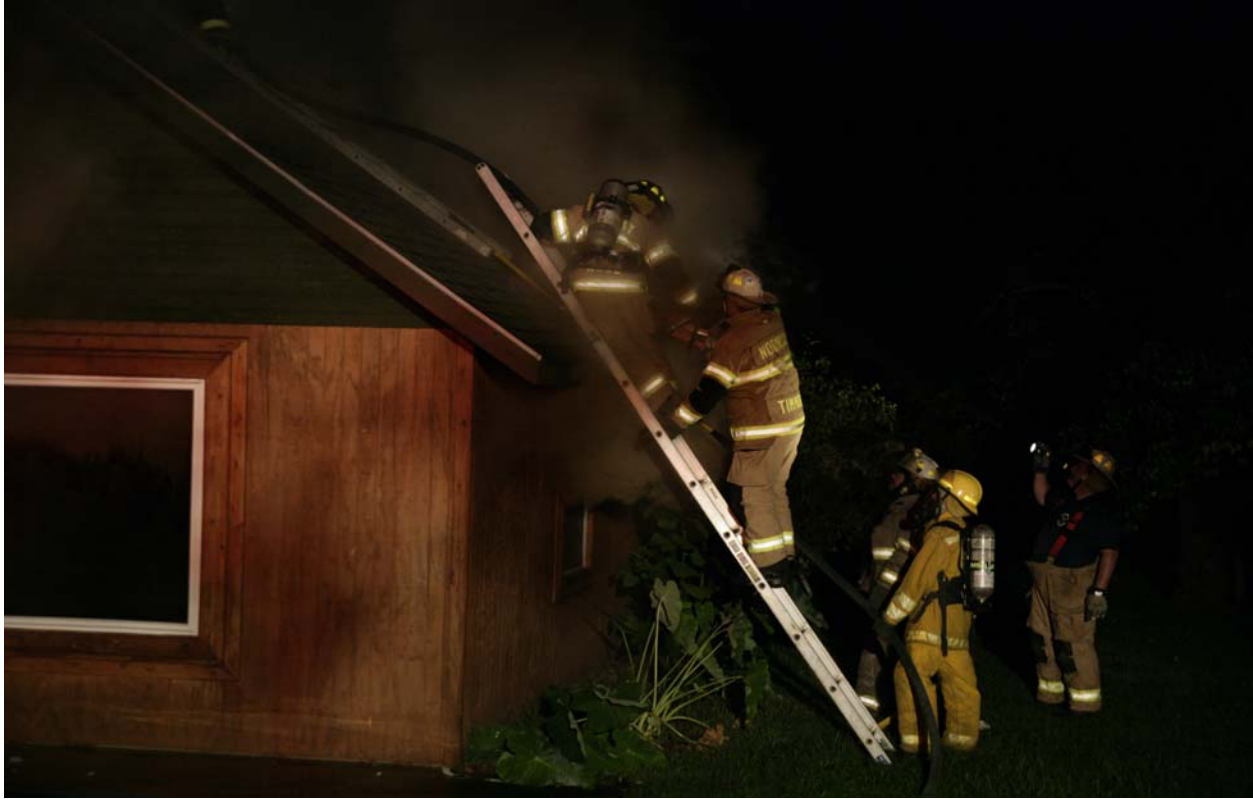
At 02:26 the safety line is on the roof as a power saw is passed up the ladder. (Photo by Bullard FD)
