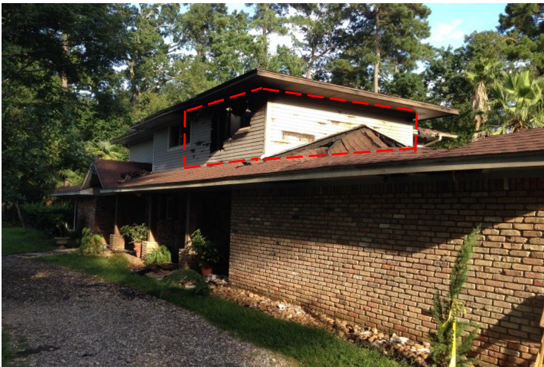
Area of void space. The garage attic opened into the void space at the garage roof peak.
