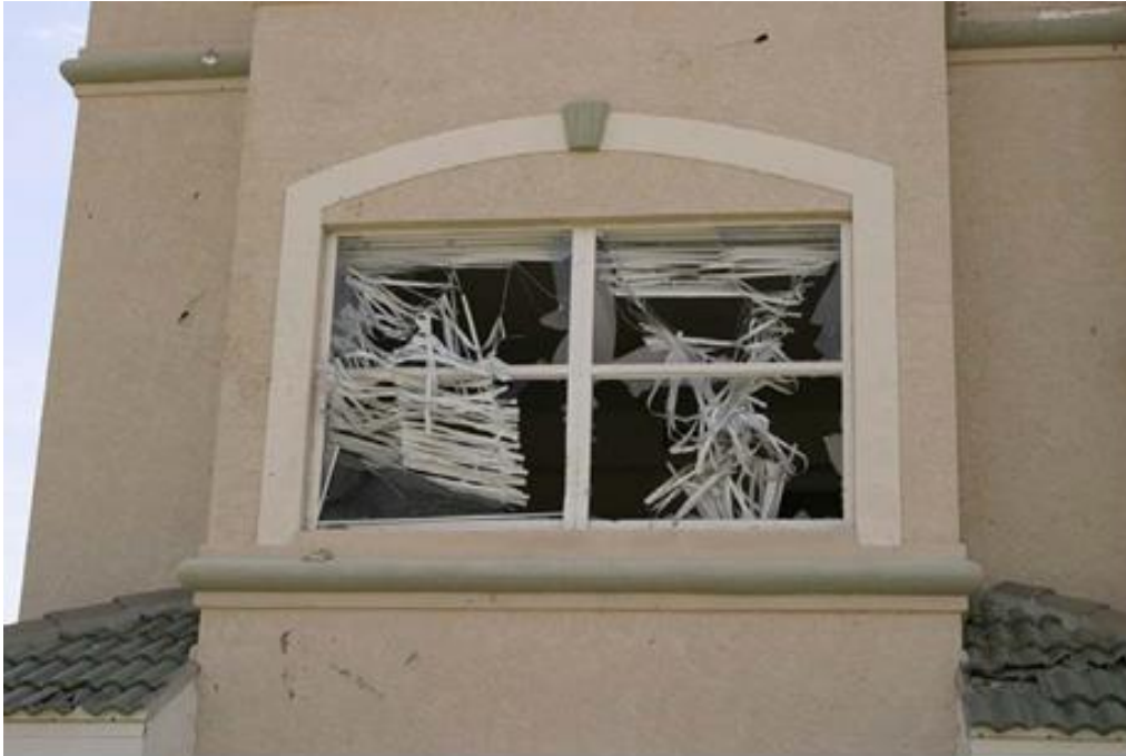
Window Glass Broken from Windborne Debris
