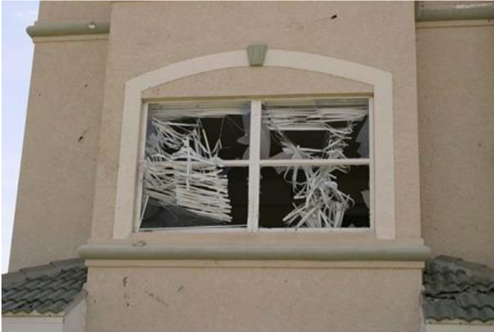
Window Glass Broken from Windborne Debris
