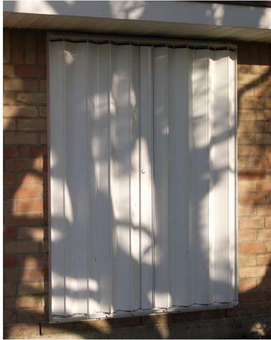
Impact Resistant Shutter System Installed Over a Window Opening
