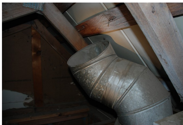
Bldg. 6 trash chute vented into the attic space. Bldg. 5 reported to be similar. (ATF Photo)
