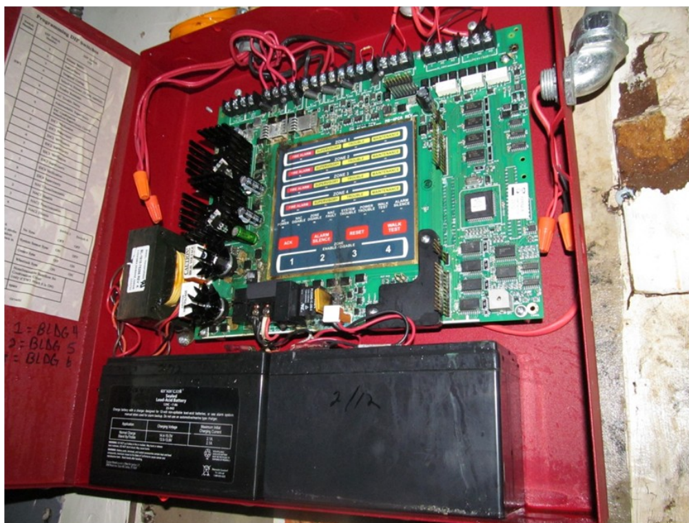
The fire alarm control panel in Building 5 was monitored by an off-premise monitoring firm
