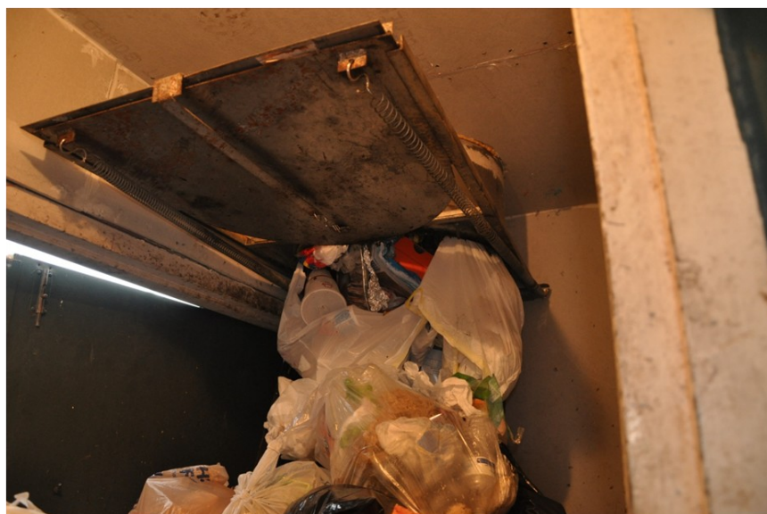
Condition of trash chute spring-loaded door at first floor in exemplar building
