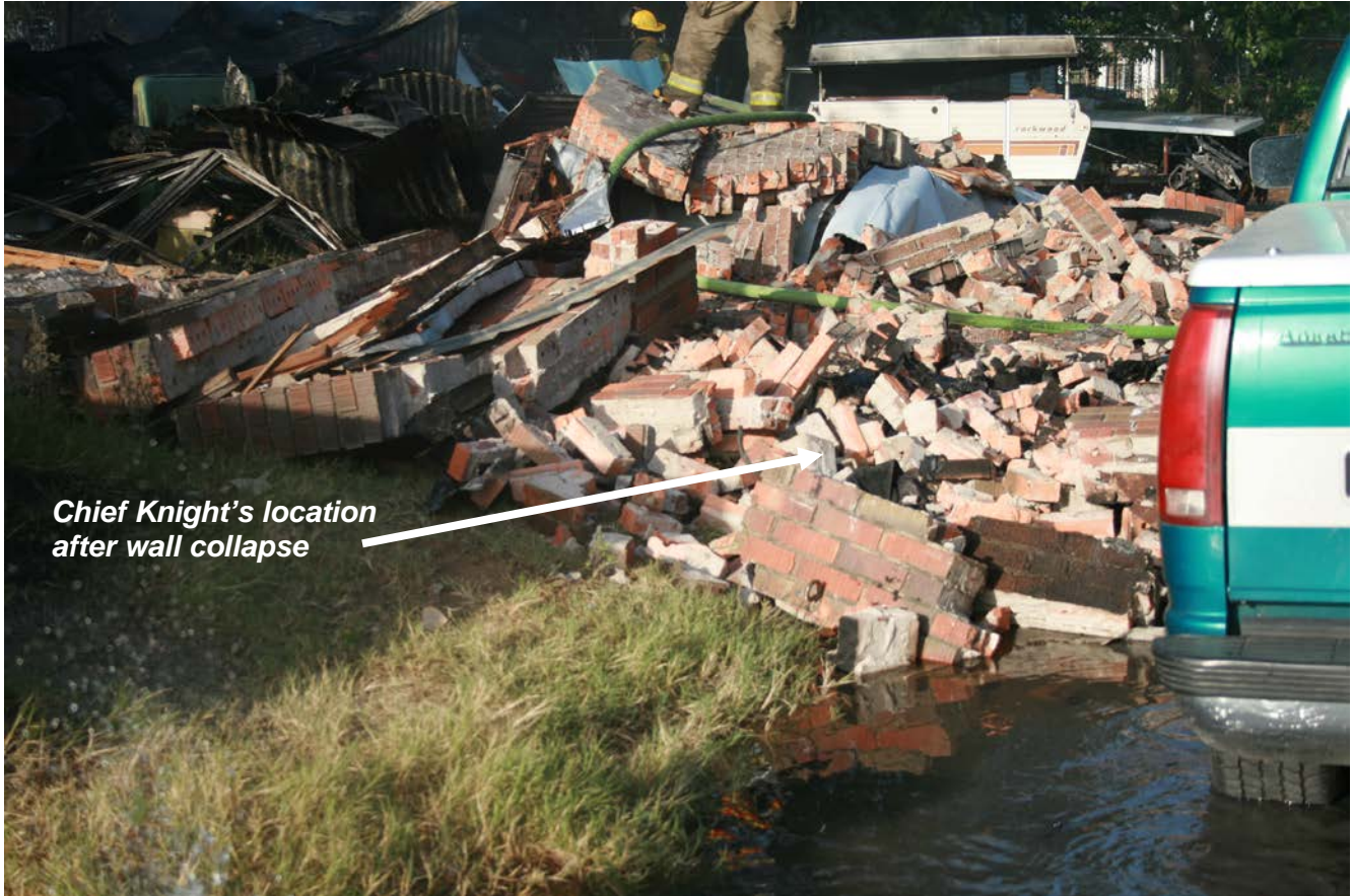
This photo shows the site of the collapse at Chief Knight's location. (Courtesy of Teague VFD)
