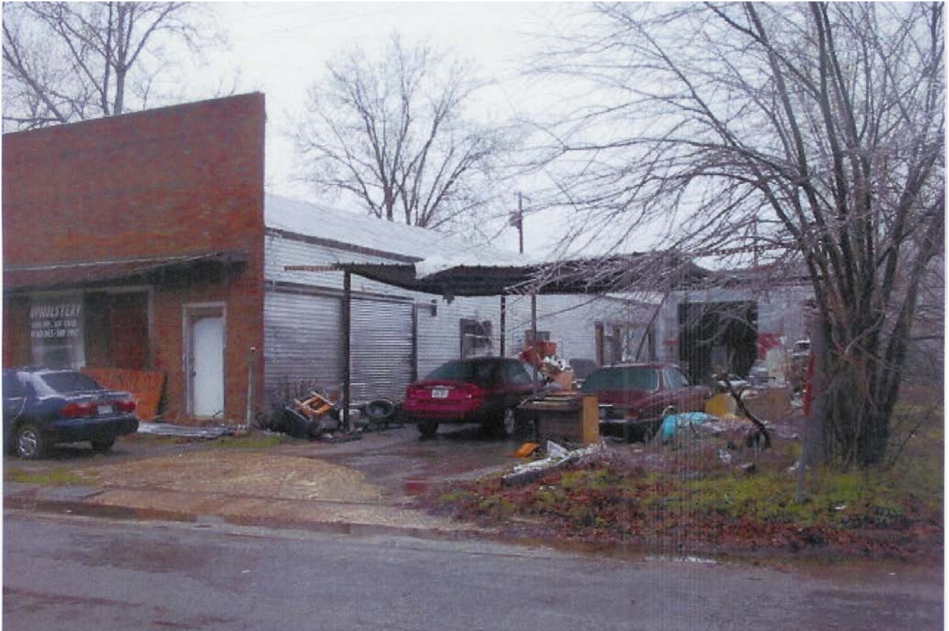
The construction type and condition of the building is shown in this 2003 photograph provided by the Freestone County Appraisal District.
