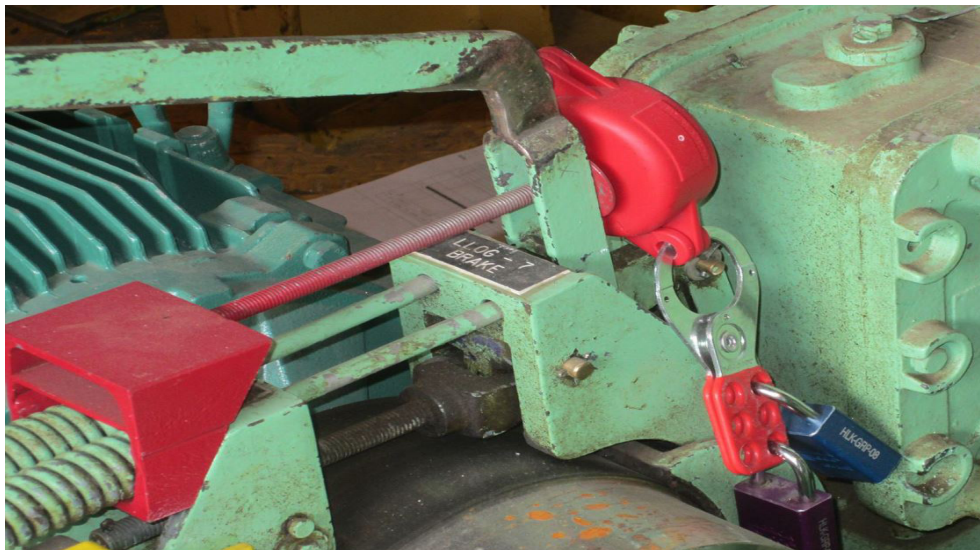
A lockout device applied to a hoist brake.
